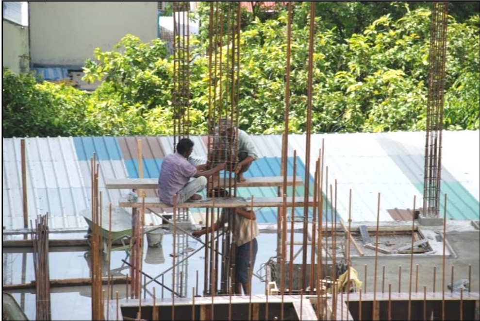
Construction workers working with no safety equipment or measures
