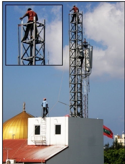
Technicians with no safety equipment or measures – a common sight in the Maldives
