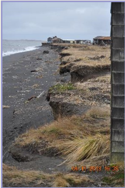
2013 erosion at Meshik site in Port Heiden (Jaelyn Christensen).
