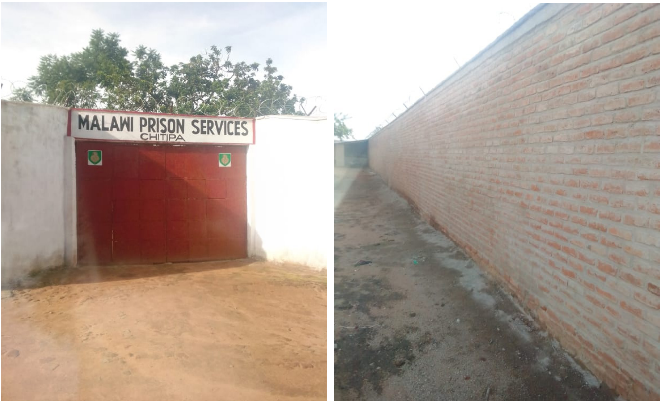
Figure 7: Picture of a new fence constructed at Chitipa Prison replacing a grass enclosure.
