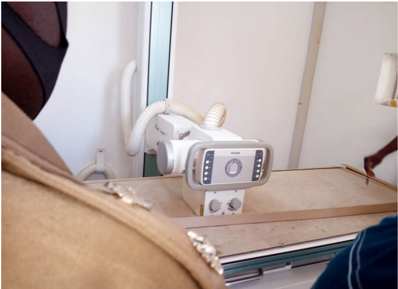
Figure 14: Inspectors appreciating the x-ray machine which had been idle since its installation at the prison.
