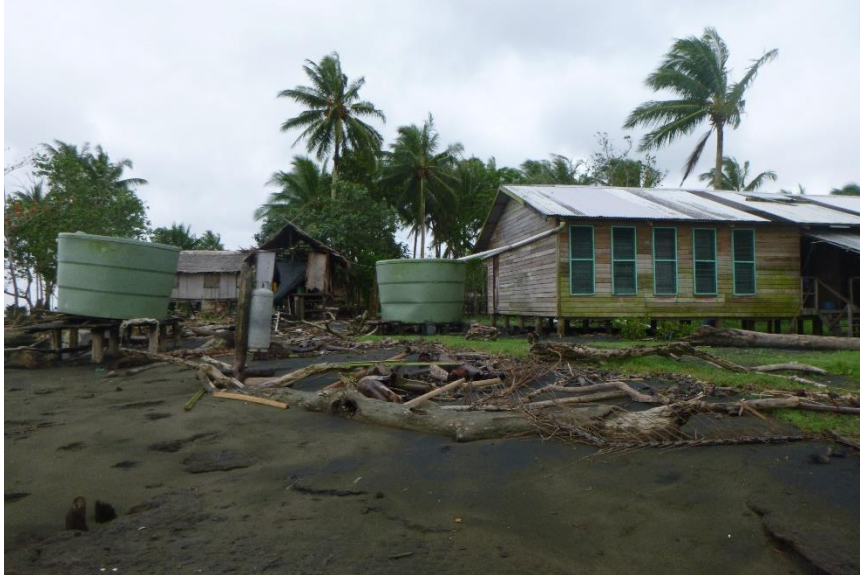
Photo 2. In 2020, the rising sea and waves destroyed two teacher’s houses and forced us to close the school and consider relocation. This is the second relocation.
