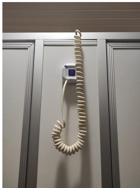
Emergency call system installed in an inconvenient position
