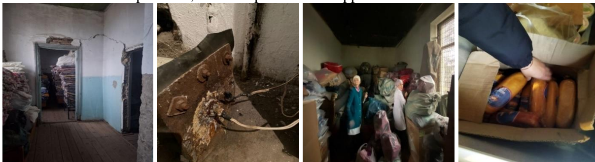
Photos 64, 65 The room is in emergency condition, bare wires
