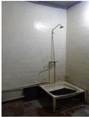
Shower room in Ekibastuz TDF
