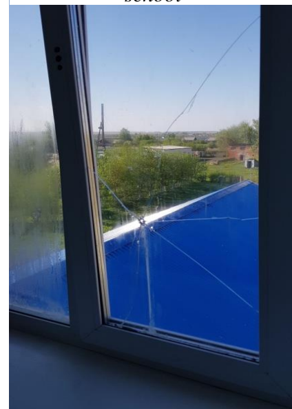
Broken windows in the Sokolovsky special boarding school
