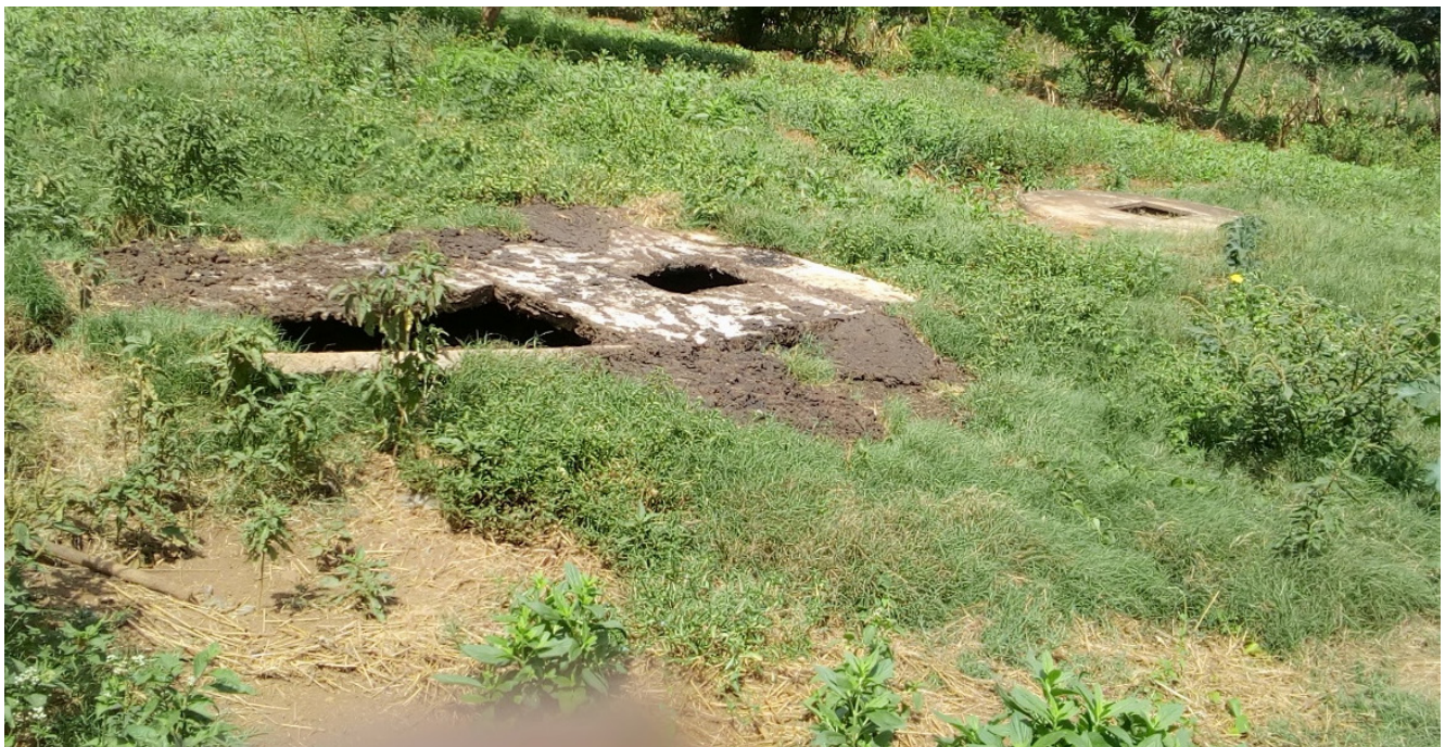
Figure 11: Septic tank at Mwanza Prison
