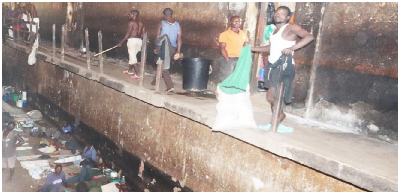
Figure 4: Dilapidated B Block at Zomba Central prison with no handrails to protect falling down from upper storey.
