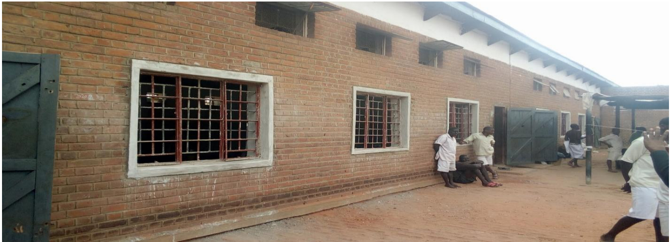
Figure 8a: Chikhwawa prison showing larger windows fitted to improve ventilation. The cells had initially had only the small windows appearing above the large windows.
