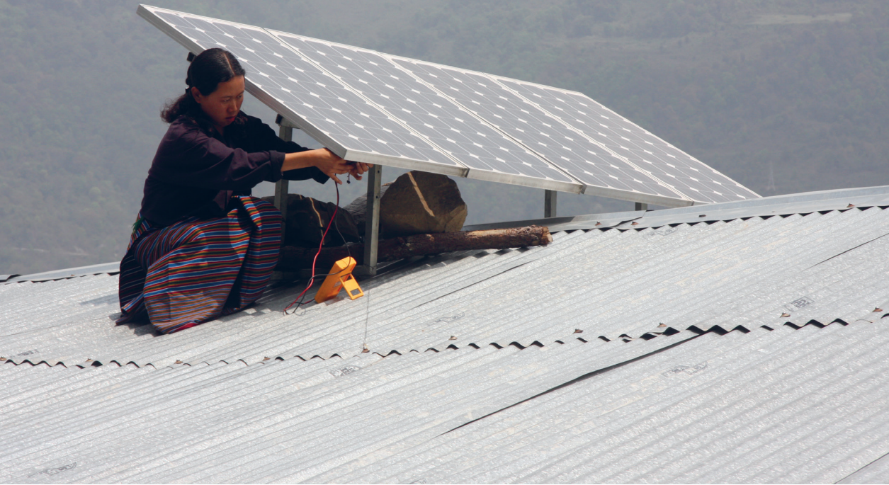
A woman installing solar panels on the roof in Bhutan. (CC BY-NC-ND 2.0 Asian Development Bank – flickr)
