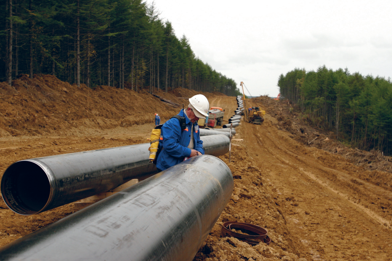
Pipeline construction and foundation work is undertaken for a gas plant and oil terminal in Russia. (© Peter Blakely – Redux/laif)
