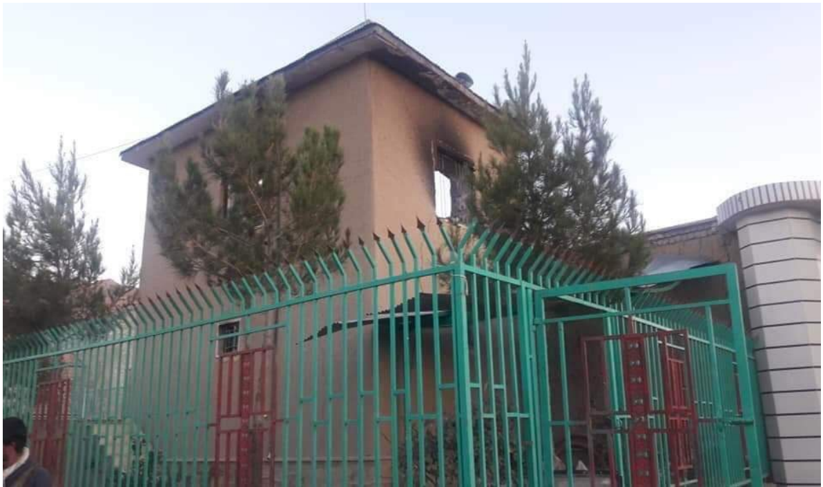
Burnt and damaged house at Hotqul area, Jaghori district, courtesy provided by Eid Mohammad Poyesh
