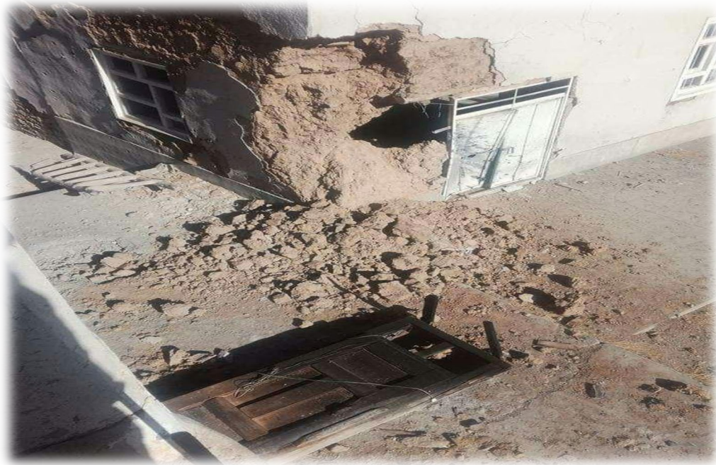
Burnt and damaged house at Malistan district, photo provided by: Bahrami
