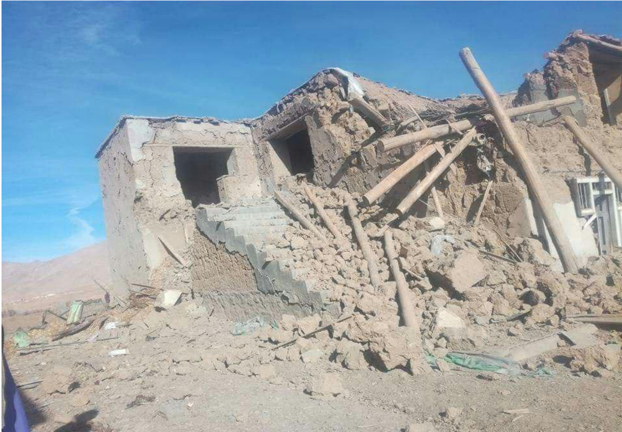
A Hazara district, where a house destroyed after the Taliban attack on November, 2018. Photo provided by Bahrami.
