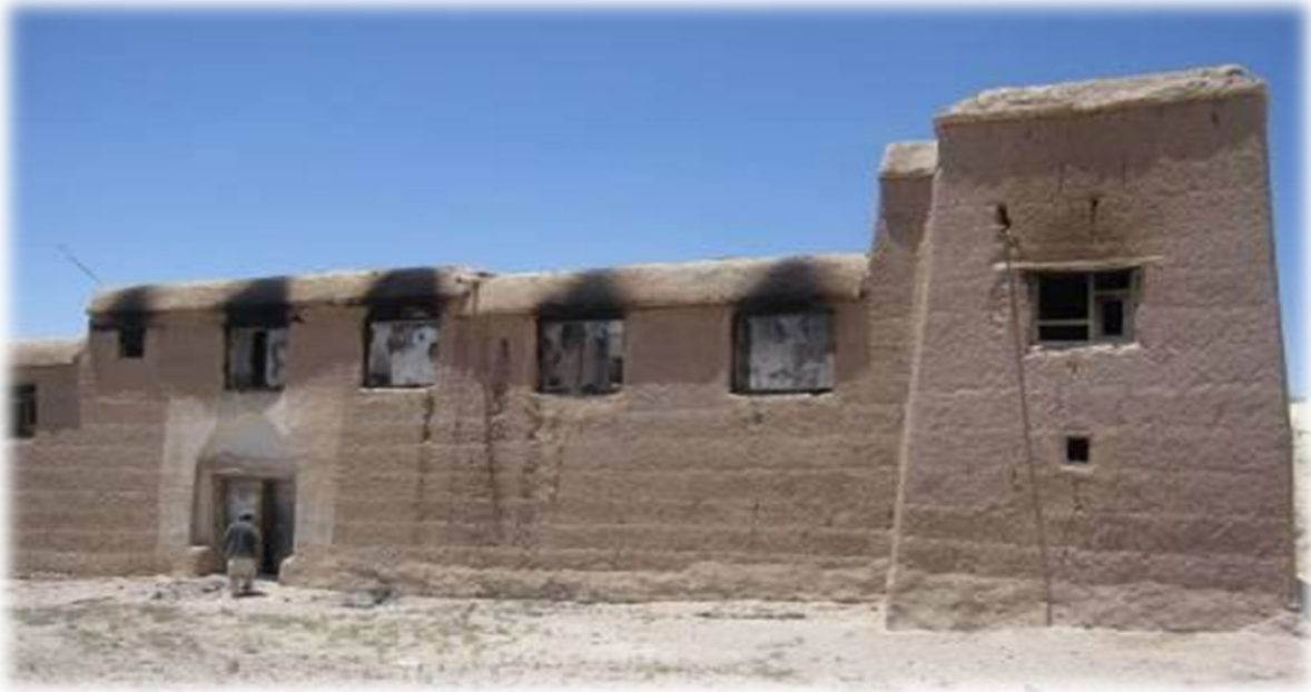
A burnt building in Nahoor District; the photo is provided by AIHRC staff.
