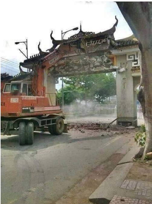
Picture 2: Destruction of gate to Preah Trapeang Province
