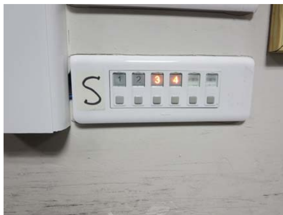
Call control board at Ilundáin, Aranguren (Navarre)
