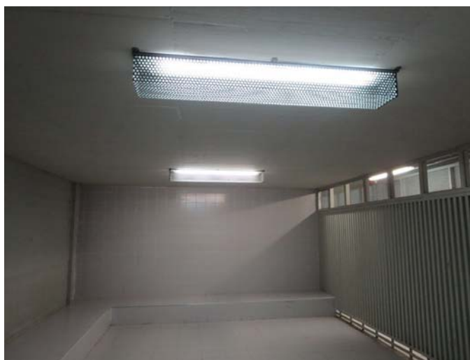
Lighting of a cell in Motril (Granada)
