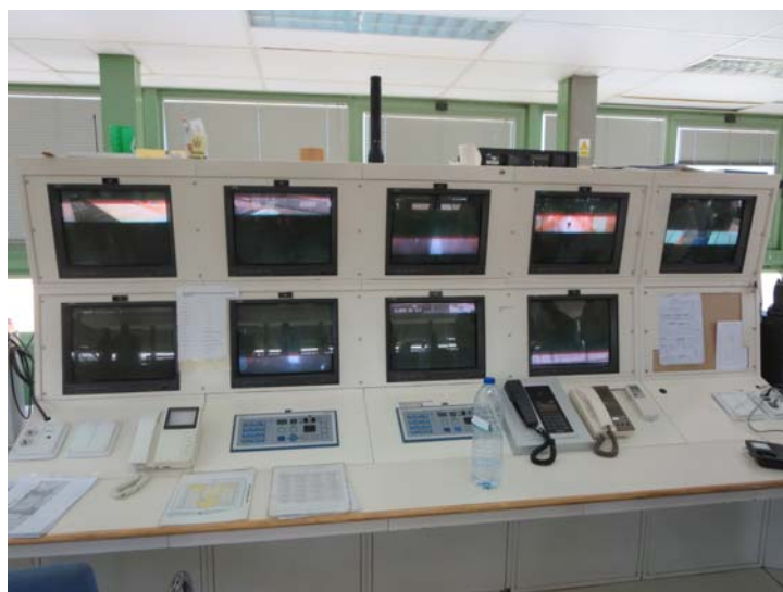
Video-surveillance system at the CP of Topas (Salamanca)
