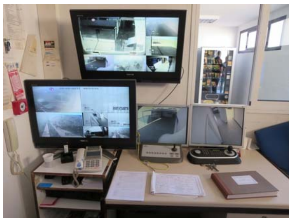
Screens to view pictures at the CIE of Tenerife
