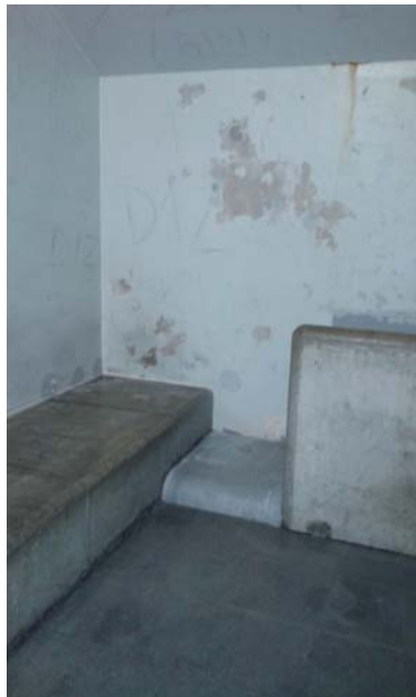
Toilets within a cell at the Police Station of the Mossos d'Esquadra of Barcelona
