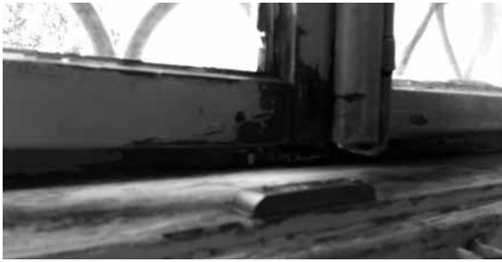
One of the windows in Ig Prison which cannot be closed.
