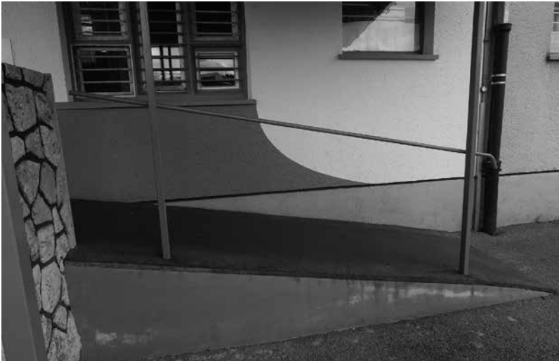
Too steep ramp in Department III of Dob Prison
