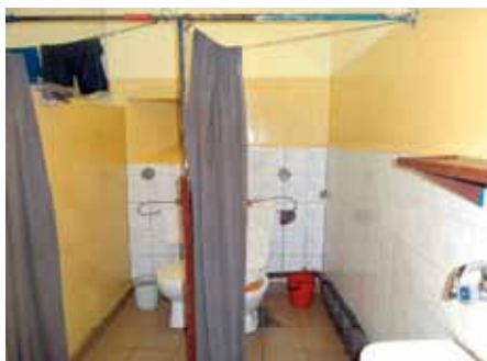
Sanitary area in a cell for 19 inmates (Pre-Trial Detention Centre in Bytom)
