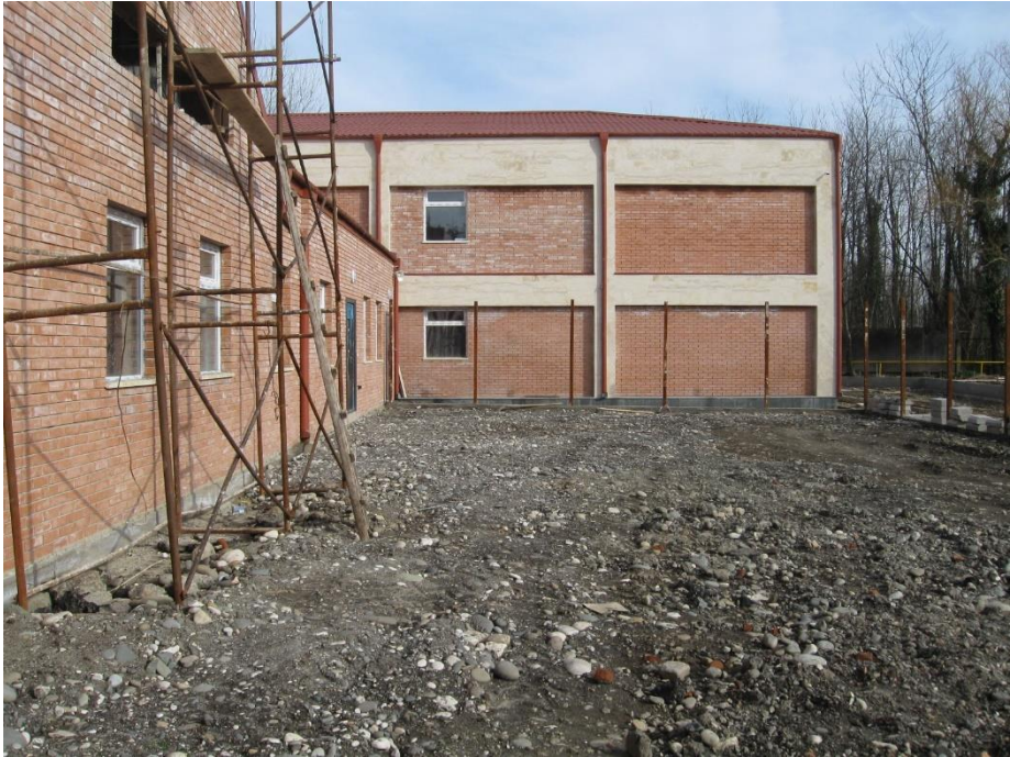
The new building of the National Center for Mental Health, where the repair works are underway
