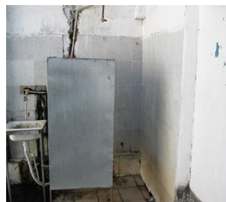
TDF of the IAB of Issyk-Ata district. Bathroom
