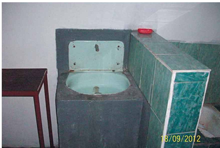
Photo: absence of faucet in the room for apprehended and detained persons, Pidvolochisk District Unit of MIA Department in Ternopil Region;
