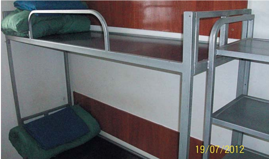
Photo: the bed railings in the room for apprehended and detained persons at Obolonsky District Unit (MIA Main Department in the City of Kyiv) do not exclude the possibility of suicide by hanging
