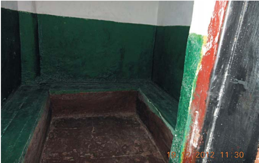
Photo: at the room for apprehended and detained persons of Tsentralny District Unit, Simferopol City Department of MIA Main Department in the Autonomous Republic of Crimea
