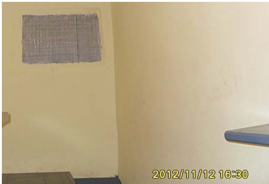
Photo: no vent at the temporary holding facility of Kovel City Unit, MIA Department in Volyn Region
