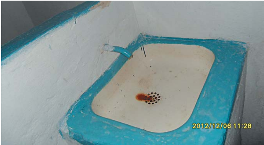
Photo: absence of faucet at the temporary holding facility of Volnovakha District Unit, MIA Main Department in Donetsk Region
