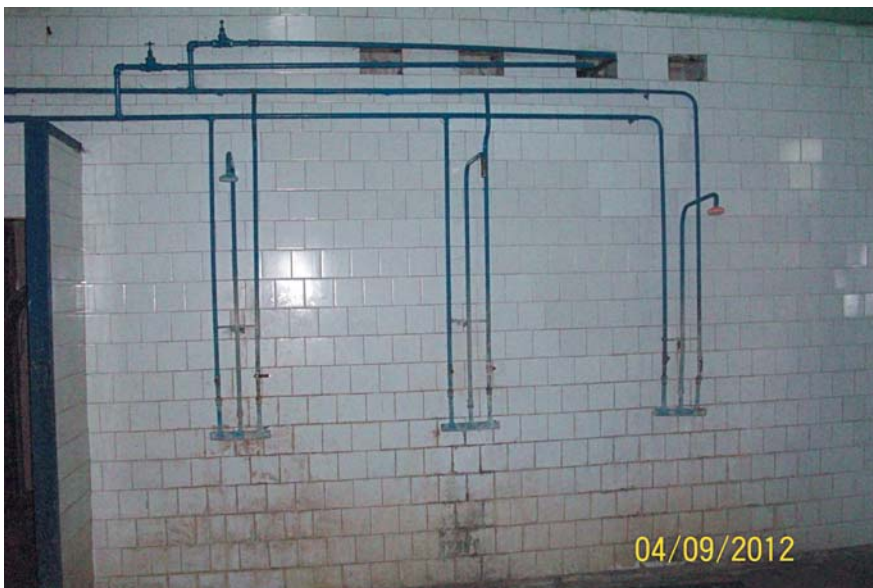
Photo: at the sanitary inspection room of the special reception center for persons under administrative arrest, MIA Main Department in the City of Kyiv: no sprinkles and poor sanitation
