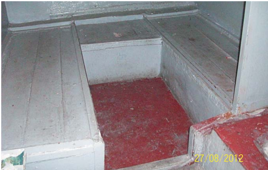
Photo: the berths at the temporary holding facility of Kotovsk City Unit of MIA Department in Odessa Region do not conform with the established size or design
