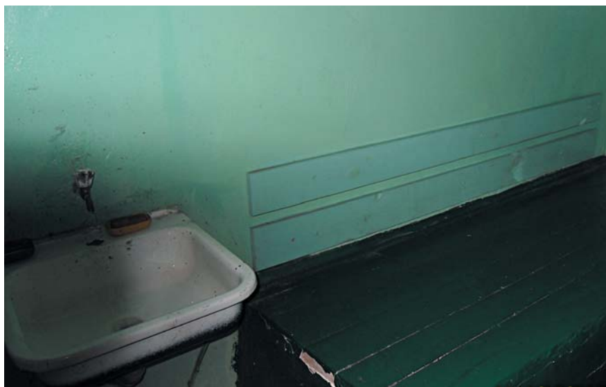
Photo: the berth at the room for apprehended and detained persons of Pechersky District Unit under MIA Main Department in the City of Kyiv has no soft protective covering and does not meet the size and design standards
