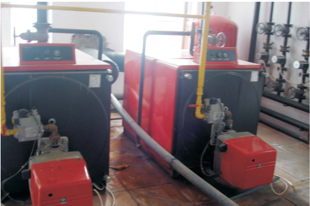
Photo 34. ME Open Special Correctional Institution for Boys. New boiler room.
